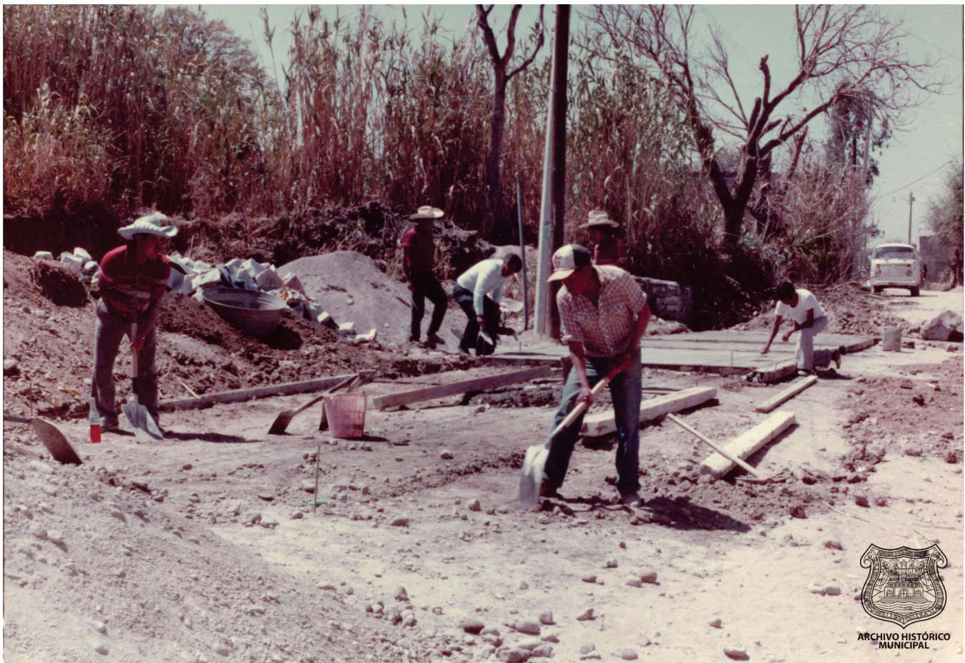
Figure 2. Urbanization of Ignacio Romero Vargas in the mid-1980s. This image shows the construction of a road, also in the background it can be observed abundant vegetation mainly composed of wild cane or giant reed ( Arundo donax ), a plant species that grows in wetlands and near rivers serving as a refuge for amphibians, birds and reptiles. Photograph courtesy of Archivo Histórico Municipal de Puebla.
